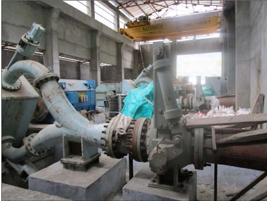
Pic-23 Crane & Other equipment in Power House
