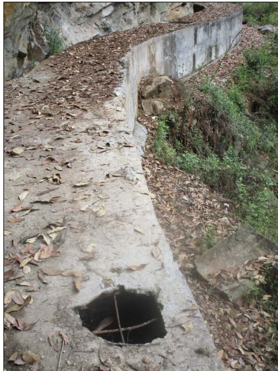
Pic-8 Damage roof of Power Channel
