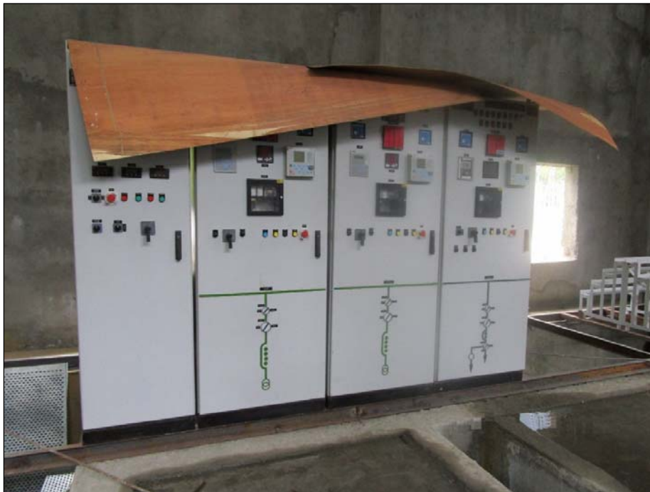
Pic-24 Control Panels in Power House
