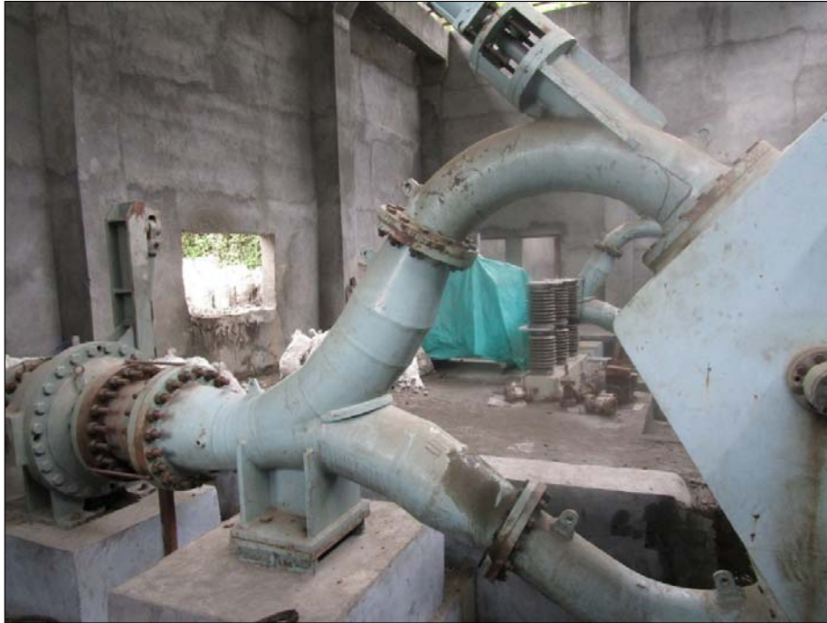
Pic-21 Pelton Turbine inside Power House
