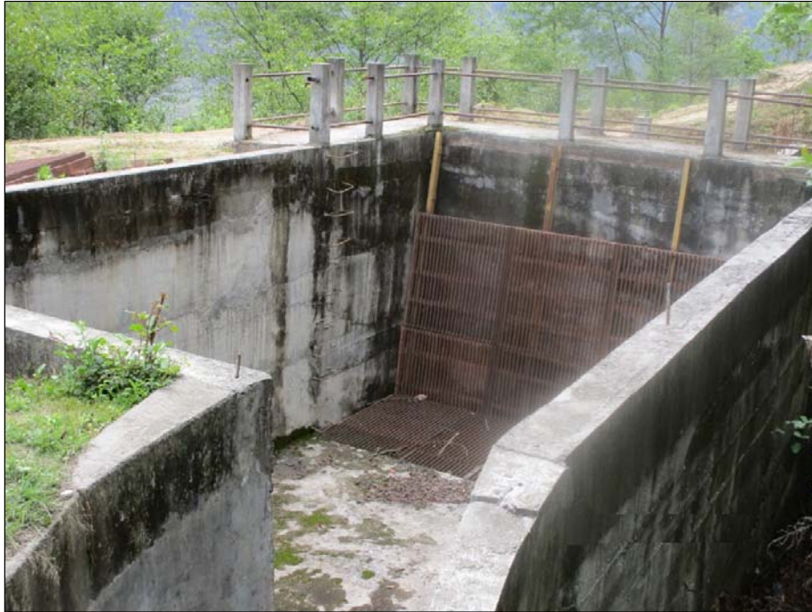
Pic-9 Forebay Tank
