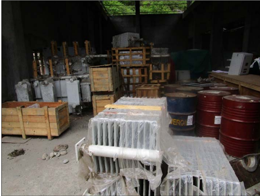
Pic-25 Equipment at site (To be installed)
