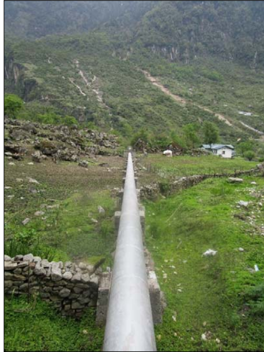
Pic-17 Penstock with supports going to Power House
