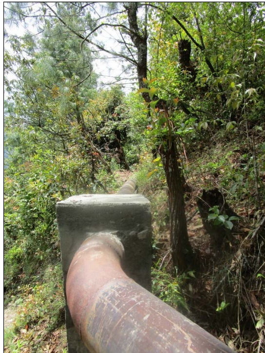
Pic-14 View of Penstock
